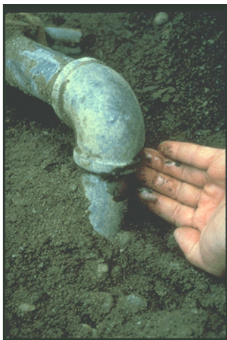
Leaking pipe from UST
